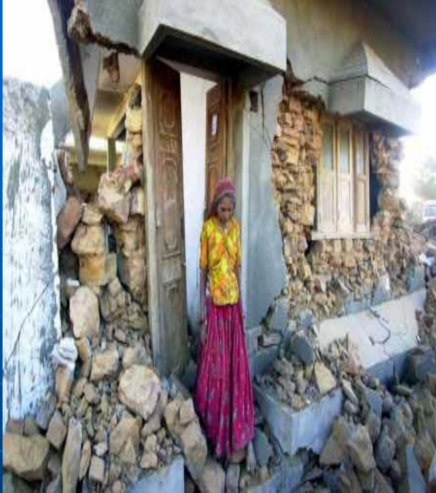
A lady standing in front of her rumbled house in Rapar, Gujarat after 2001 earthquake
